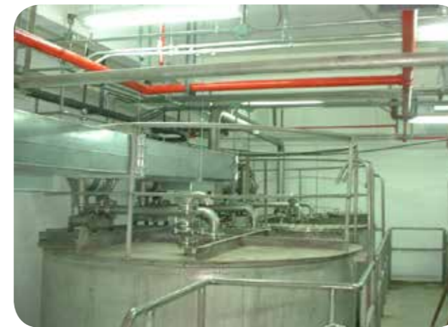
Storage Tank of Liquid Waste
