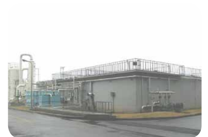
Domestic Sewage Treatment Facility
