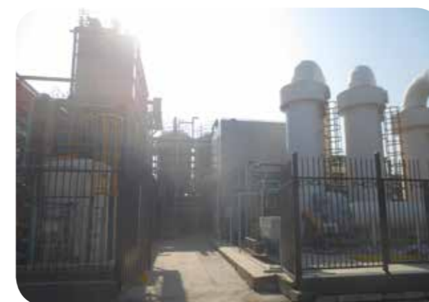
Ammonia Nitrogen Wastewater Treatment Facility
