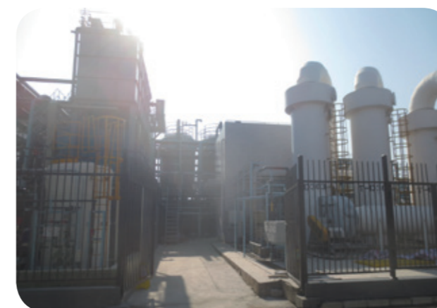
Ammonia Nitrogen Wastewater Treatment Facility
